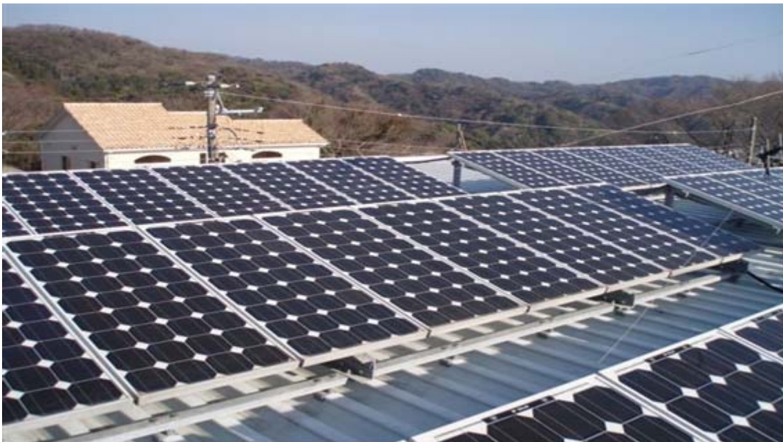
Figure 8 An example of solar power generation (PV) set-up
