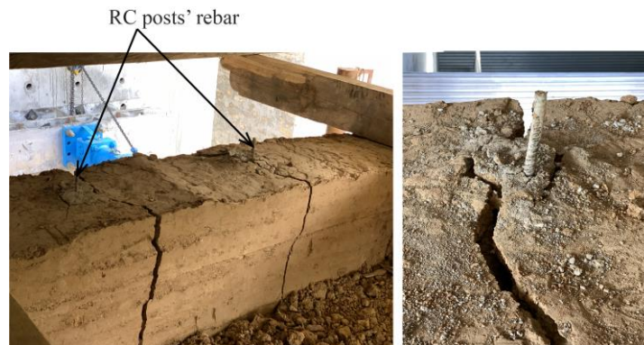
Figure 5.45 Cracks near RC posts of New-RE-SHORT.
