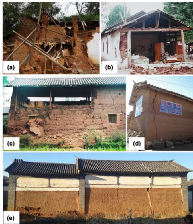
Figure 2.6 Damages observed in rammed earth houses: (a) structural collapse; (b) gable wall fall-over; (c) longitudinal wall fall-over, (d) vertical corner crack; (e) Crack at loading point [13].
