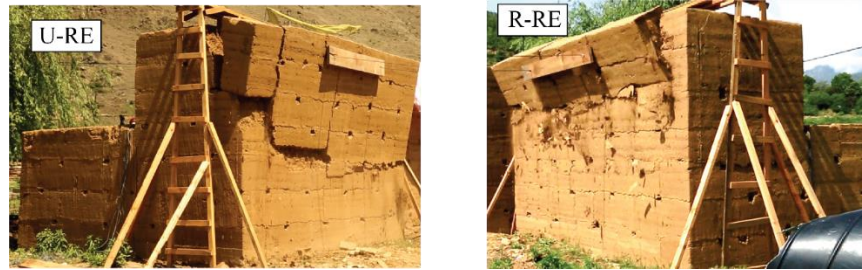
Figure 4.54 Damage of U-RE and R-RE specimens during “Pull-down-1” test.
